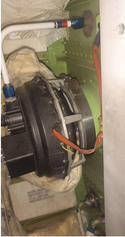
Figure 2 – VIEW SHOWING INSULATION STUCK IN VALVE. NOTE PROPER INSTALLATION OF INSULATION IS REQUIRED TO PREVENT THIS PROBLEM.
