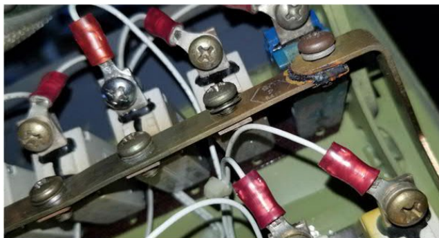
Indication of burning due to arcing of loose (under torqued) bus bar connection.
